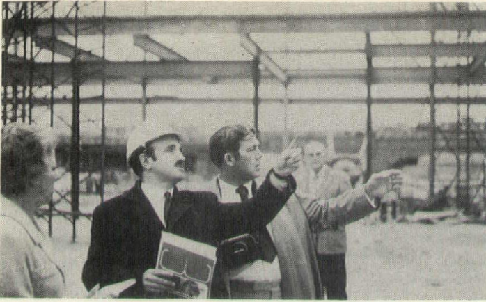
Mr. Roy Lewis, Section Engineer, Sir Robert McAlpine & Sons, London, England, points out feature to Aubrey Bass, Bass Construction Co., Inc., Richmond (current President of Virginia Branch AGC). Looking on are Mrs. James F. Duckhardt (wife of Virginia Branch AGC Executive Director), Richmond, (left), and Glen Barker, Barker Construction Co., Inc., Richmond (background).
