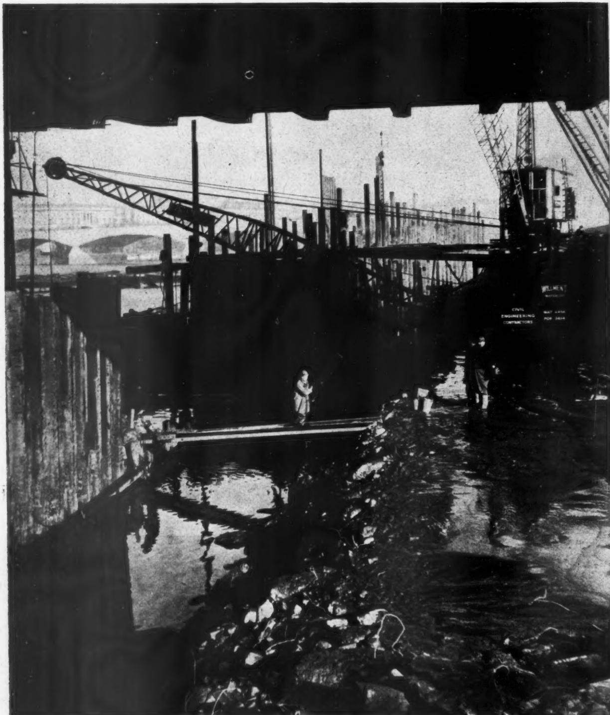
Above is shown the line of the steel cofferdam, rammed home into the river bed, near Hungerford Bridge. The work is being done by Richard Costain, Ltd., at a cost of £250,000.
