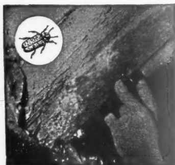
A rafter in the roof of Chichester Cathedral showing damage by the Death Watch Beetle.
