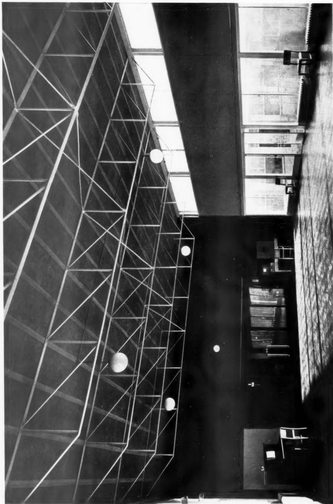
The light steel trusses with lattice bracing support a roof of woodwork slabs.
