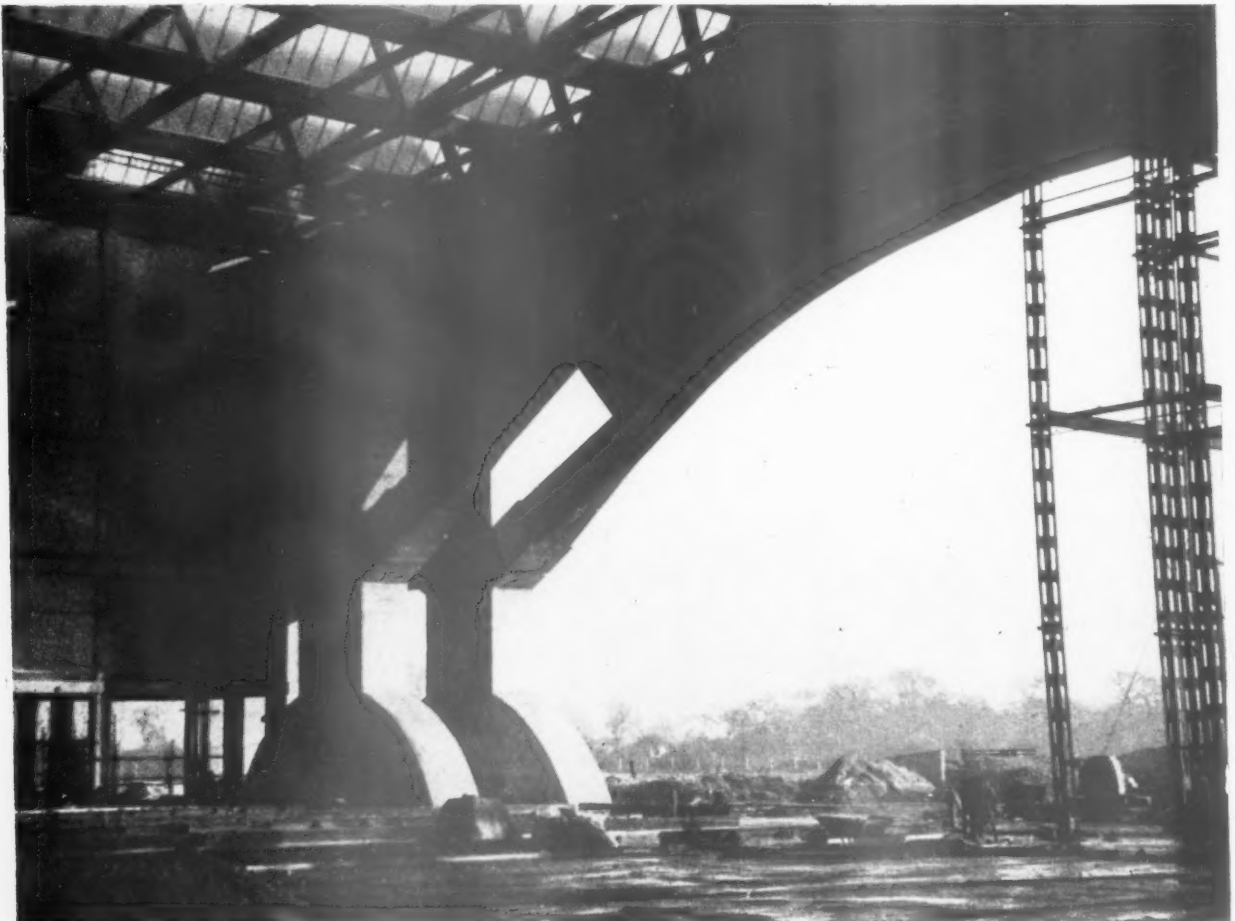
This BOAC headquarters under construction at London Airport was designed by Sir Owen Williams and Partners.
