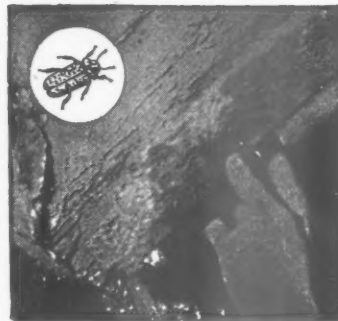
A rafter in the roof of Chichester Cathedral showing damage by the Death Watch Beetle.
