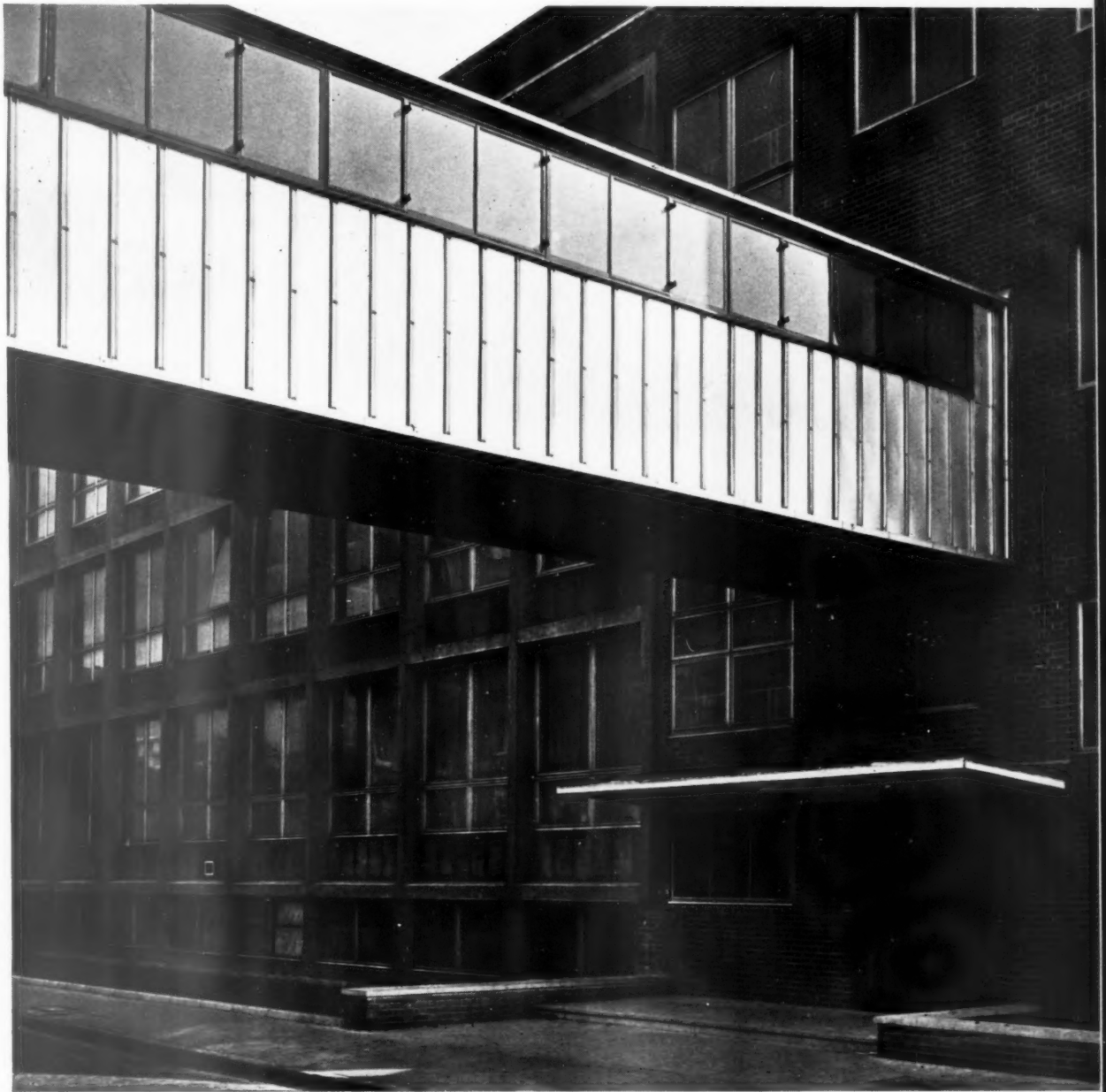
The aluminium cladding conceals the steel structure of the bridge and the sloping floor between the old and new buildings.
