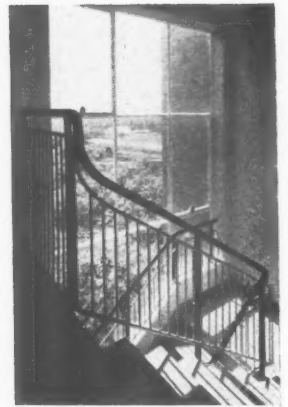
Left, block 1 from the south-west. On the right the south staircase window. Above, staircase in this block, from the eleventh floor.
