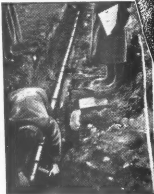
We illustrate below a photograph taken at ALDERMASTON during a recent large scale installation.
