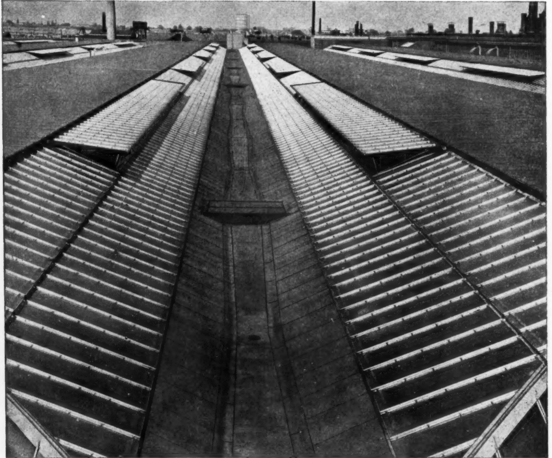
Roof of new assembly shop at Daimler Radford Works. Architects: Wood & Kendrick & Williams, F.F.R.I.B.A. Chartered Architects.
