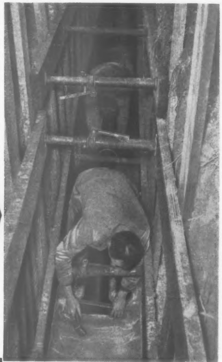
The photograph shows 6" Temple Tube being laid in the extremely difficult condition of a flooded trench, at the Caravan Site, WOODLANDS PARK ROAD, WHITE WALTHAM, NR. MAIDENHEAD, BERKS. (SURVEYOR: A. MANDEVILLE, B.sc., A.M.I., MUN.E.) (CONTRACTORS: POWELL BROS. (Maidenhead) LTD.)
