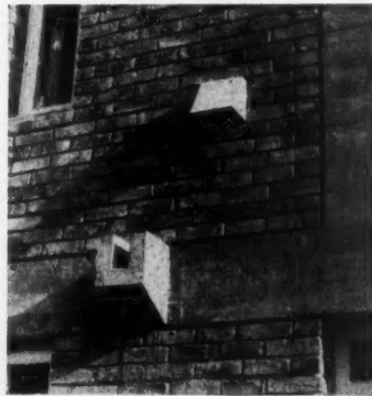
Brick and Concrete at Ham; a detail of wall, floor-slab, ventilator and gargoyle from a new flatted development at Ham Common by James Stirling and James Gowan.
