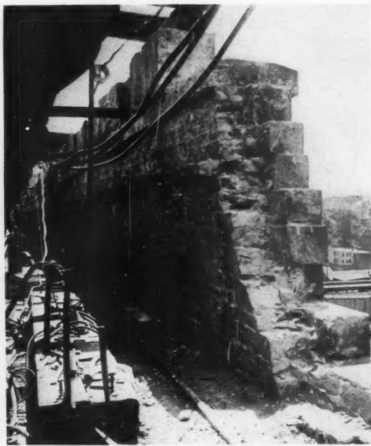
PARAPET WALL OF 1861 REMOVED AND PARAPET OF 1848 BROKEN AWAY. MASONRY WAS ASHLAR GRANITE BACKED UP WITH ASHLAR RUBBLE LAID IN NATURAL CEMENT
