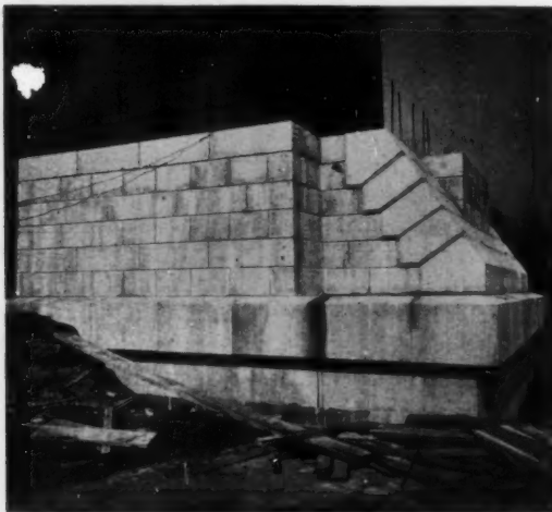
SKEWBACK ON OLD PIER TO RECEIVE STEEL ARCH. MASONRY IS SAME TYPE AS OLD
