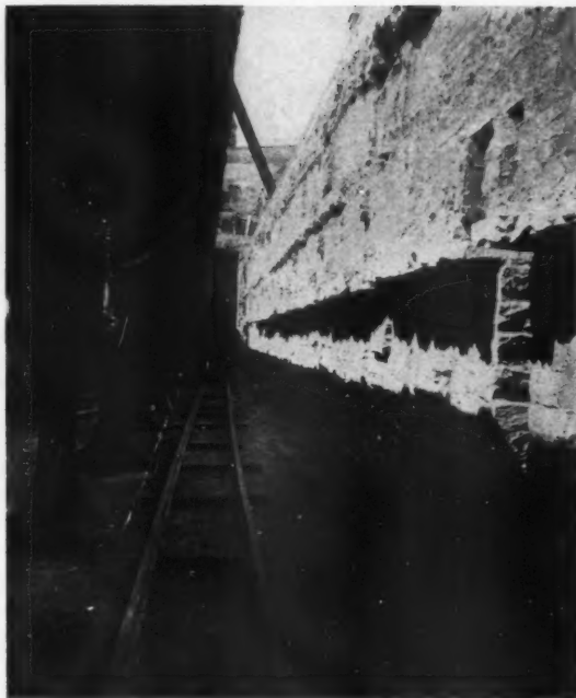
AQUEDUCT PIPE AS CARRIED WITHIN TRENCH. NOTE FLOOD DRAINAGE NICHE AT RIGHT AND LEDGE MARKING PARAPET AS INCREASED IN HEIGHT IN 1861
