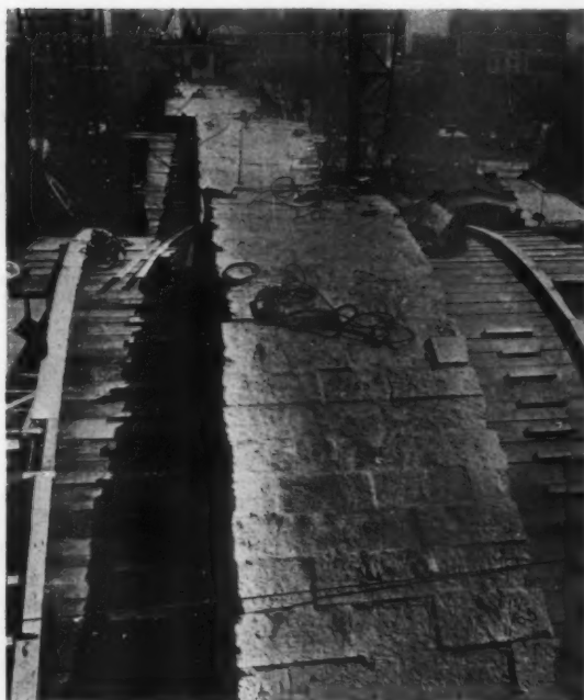
WEIGHT OF AQUEDUCT WAS DISTRIBUTED TO ARCHES BY A SERIES OF LONGITUDINAL WALLS. NOTE INSULATING WALLS AND CONSTRUCTION OF TRENCH ROOF. CONCRETE DIAPHRAGM INSTALLED TO SECURE RIGIDITY DURING RECONSTRUCTION
