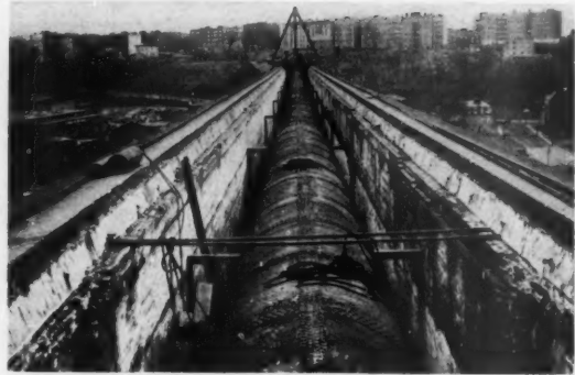
AQUEDUCT TRENCH SHOWING 90 1/2 INCH DIAMETER PIPE, CAPACITY 90 MILLION GALLONS PER DAY. DOUBLE WALLS USED TO INSULATE PIPES
