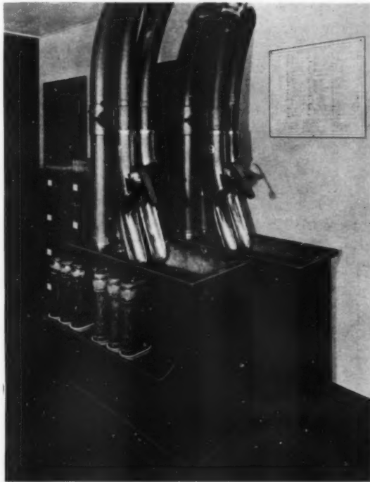
TYPICAL OUT-STATION TERMINAL AND CABINET OF PNEUMATIC TUBE CARRIER SYSTEM. EACH OUT-STATION CONSISTS OF A RECEIVING AND DISPATCHING TERMINAL
