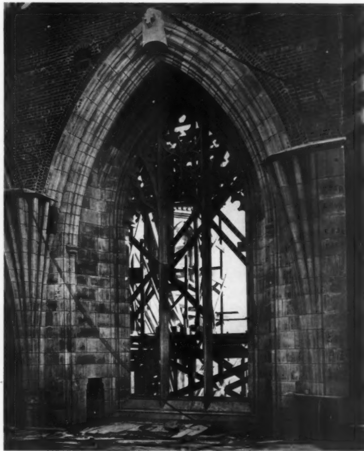
TYPICAL CHOIR CLERESTORY WINDOW WASHINGTON CATHEDRAL. WASHINGTON, D. C. FROHMAN, ROBB & LITTLE, ASSOCIATED ARCHITECTS
