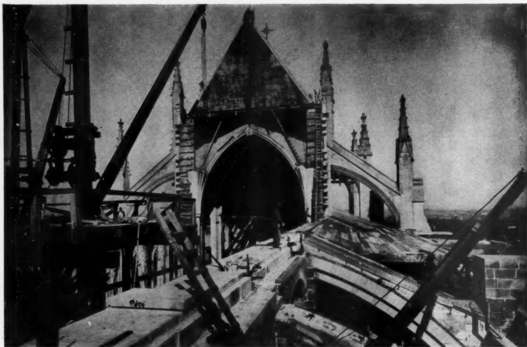
Above: GENERAL VIEW FROM SOUTHWEST SHOWING CLERESTORY OF CHOIR IN COURSE OF CONSTRUCTION
