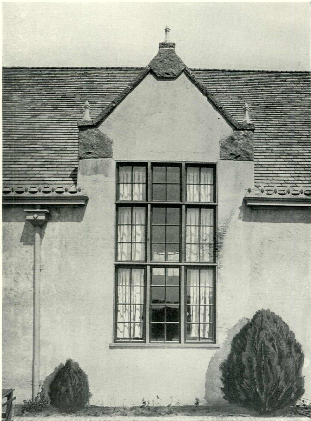
Detail of Terrace Elevation THE SOUTHERN PINES COUNTRY CLUB, SOUTHERN PINES, NORTH CAROLINA Aymar Embury II, Architect
