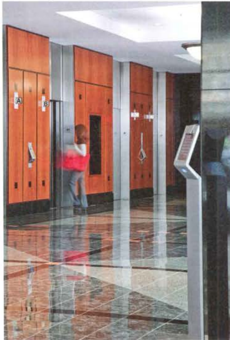
Computer-based elevator destination control systems allow users to indicate their destination before entering the car.
