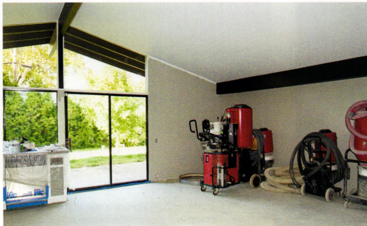
(LEFT) BE FULLY PREPARED TO MOVE OUT OF YOUR HOME IF YOU'RE CONSIDERING CONCRETE FLOORS. HEAVY MACHINERY, FINE DUST AND ACCESS TO EVERY INCH OF THE SLAB ARE ALL PART OF THE PROCESS.
