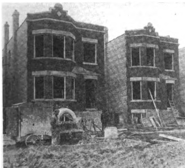
Fig. 1—Showing the Charging Side of the Mixer with Mortar Box and Sand in the Foreground
