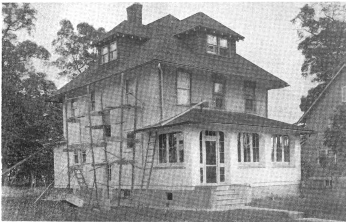
The Work in Progress—Note the Contrast Between the Renewed Surfaces of the Enclosed Porch and Those of the Front of the House Above the Porch Roof Which Have Not Been Treated
