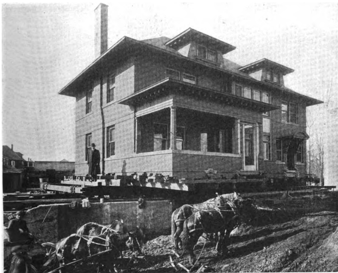
FRONT VIEW OF TWO-STORY BRICK HOUSE AS IT APPEARED AFTER IT HAD BEEN MOVED FROM ITS FOUNDATION
