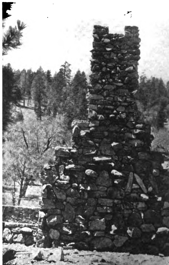
Fig. 5—Fireplace and Chimney of the Lodge as It Appeared in Process of Construction
