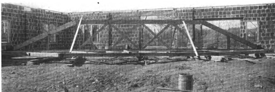
FIG. 1—GENERAL APPEARANCE OF ONE OF THE TRUSSES TOGETHER WITH A TOP VIEW
