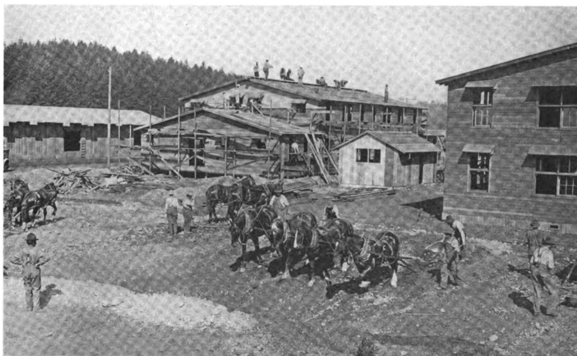
Appearance of a Two Hundred Men Barracks, Bath House and Lavatory and a Warehouse During Process of Construction
