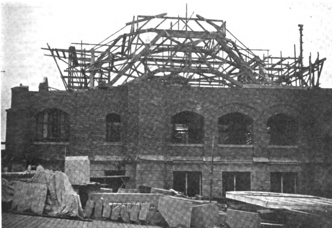
A VIEW OF SOME OF THE UNCOMPLETED FRAMING OF THE CHURCH DOME
