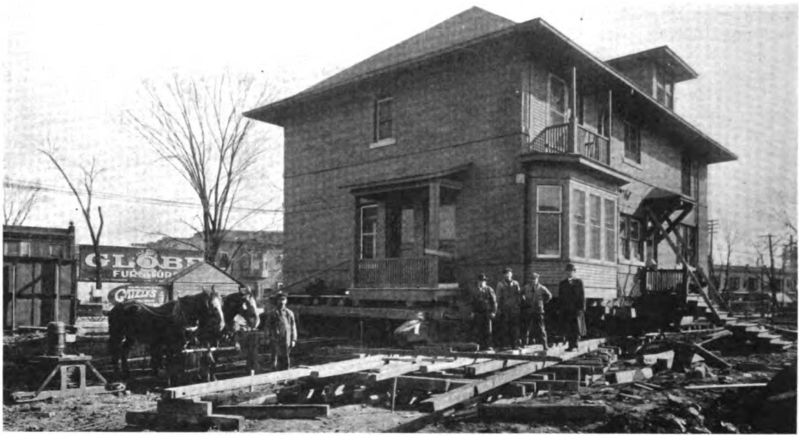
REAR VIEW OF BRICK HOUSE AS IT APPEARED DURING THE PROCESS OF TURNING
