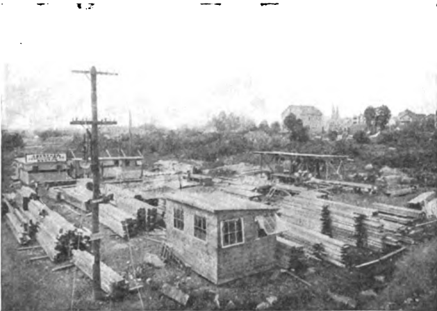
Picture of a Building Operation Showing the Distribution of the Materials, Offices, Tool Shed, Saw Mill, Etc.
