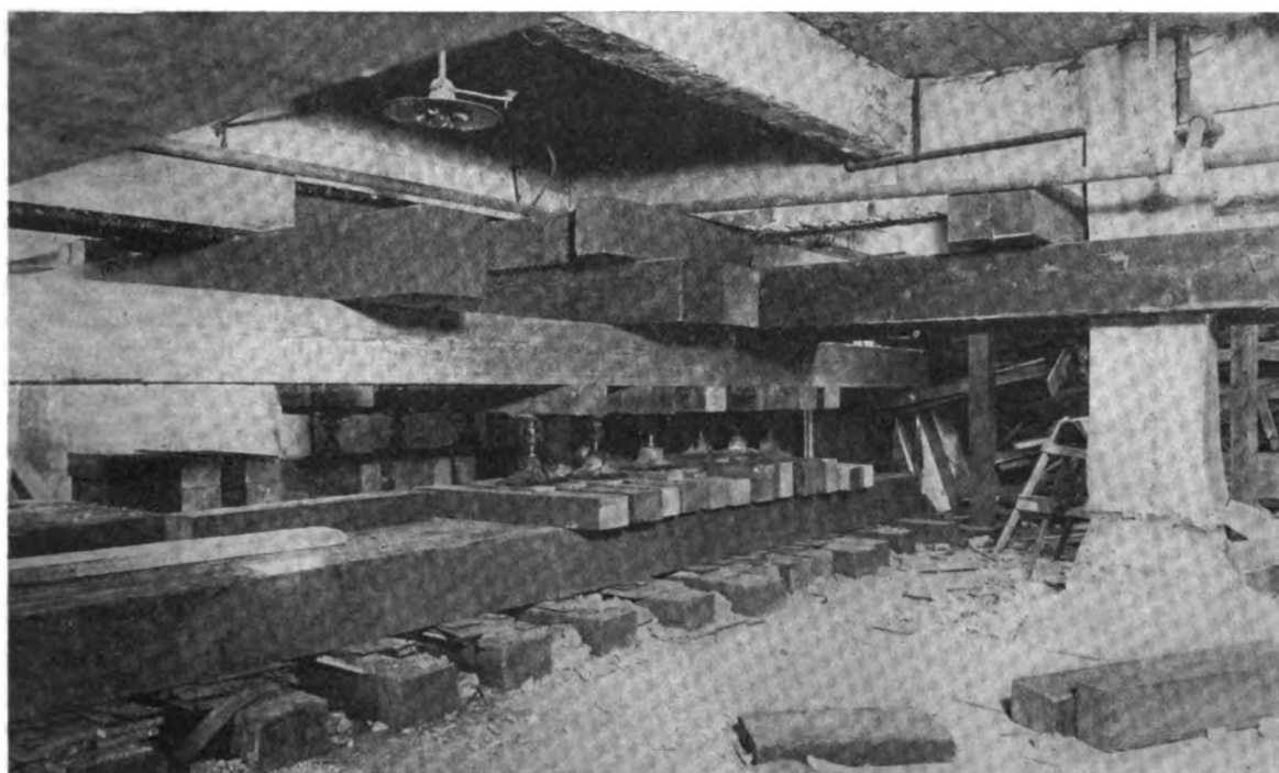
FIG. 1—THE TIMBER WORK AND SCREWS AROUND ONE OF THE CENTER COLUMNS OF THE BUILDING READY FOR LIFTING
