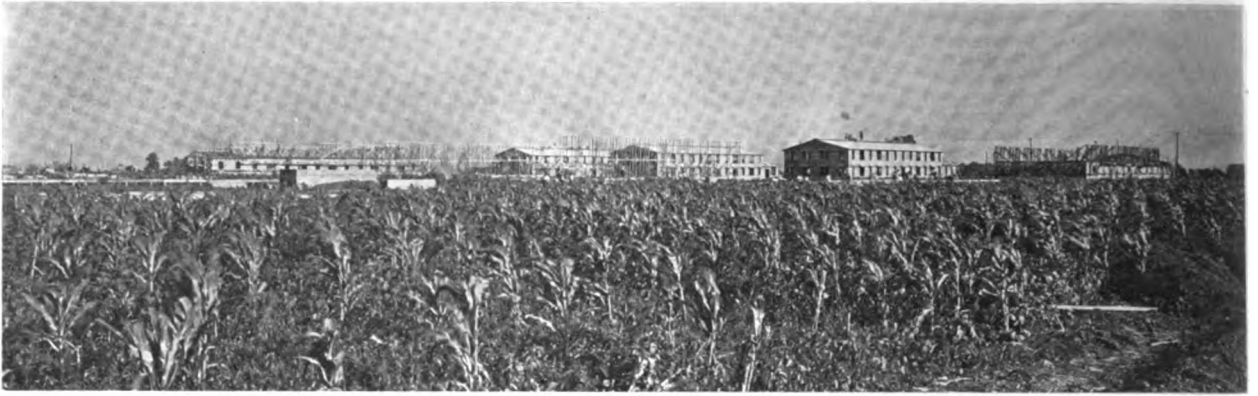
Glimpse of a Few of the Barracks Under Construction Near Louisville. In Front of the Cornfield and at the Extreme Right Is Seen the Path of the Temporary Water Main
