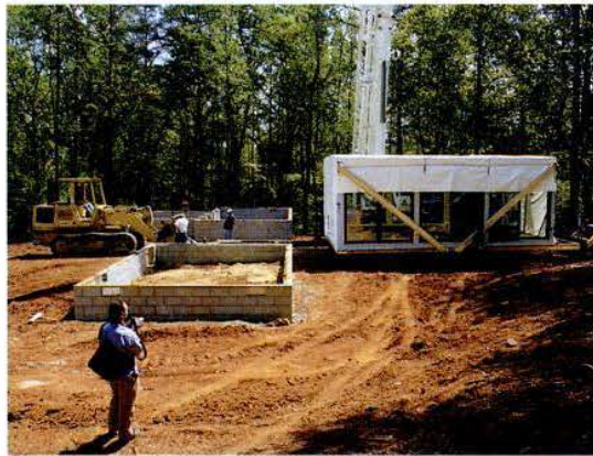
Clockwise from far left: Trucks make their way up the newly created Beech Hill Road with the modules; homeowner Nathan Wiener documents the process; modules are lowered onto the foundation.
