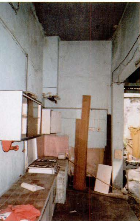
Ian and Yeo's house was uninhabitable when they purchased it in 2002. Three months later, the roof caved in. The translation of the sign above the door of the couple's renovated house (right) is "peace." Once inside, visitors are greeted by three ten-foot-tall hand-carved antique panel doors.
