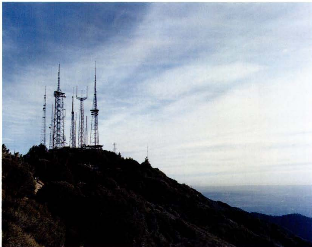
These cell phone masts atop Mt. Wilson (above), northeast of Pasadena, are the region's major relay point for police, fire, and civilian communications. i p. 238
