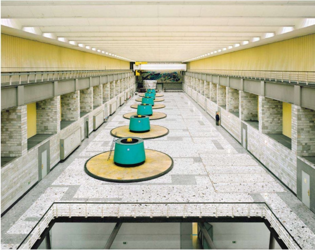
8. Engine room, La Bâthie power plant
