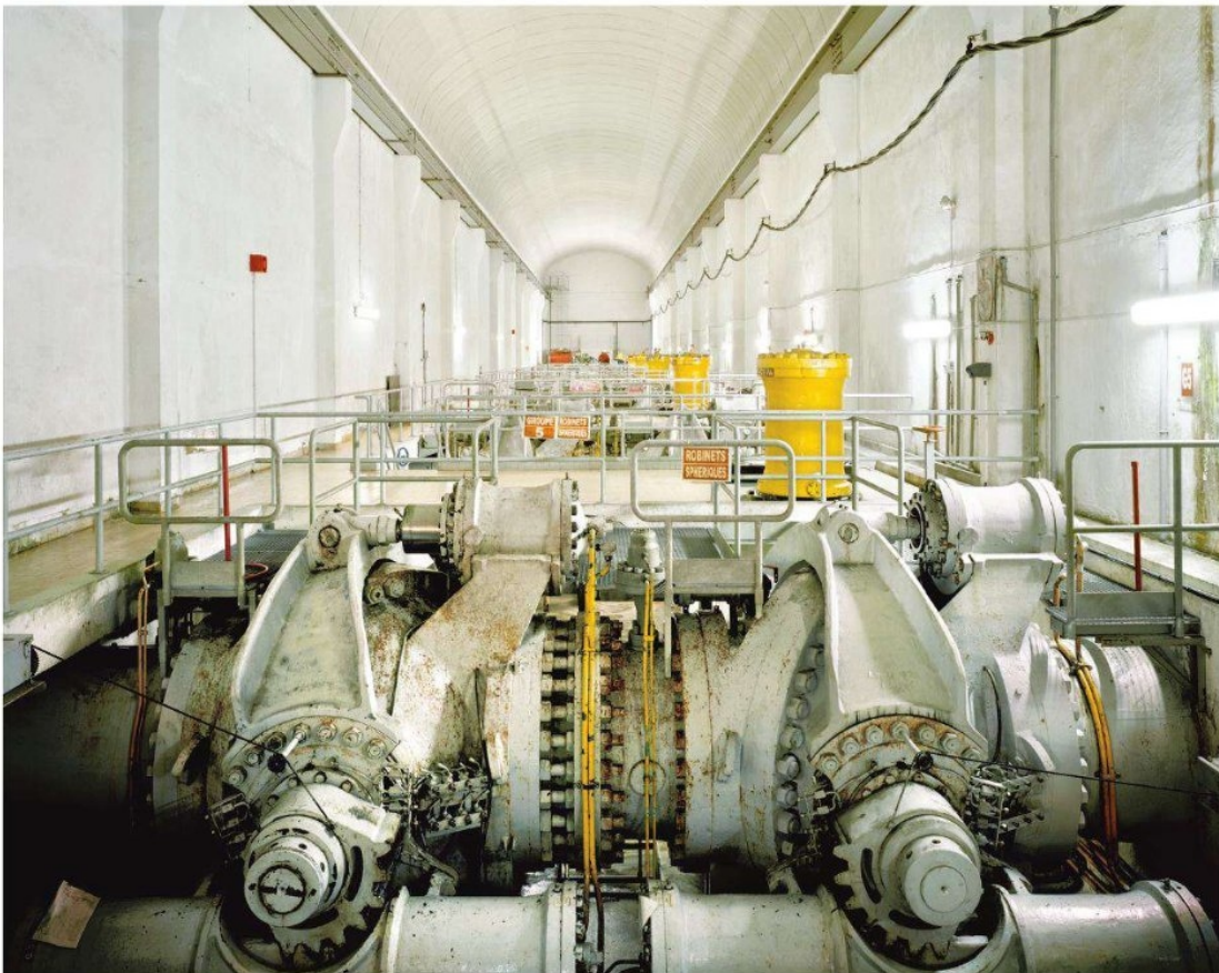
9. Valve room at the foot of the penstock, La Bâthie power plant
