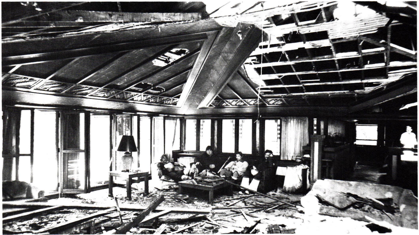
Coonley House interior looking southwest shortly after the blaze was extinguished by the fine work of Riverside's volunteer fire department. Some of them are shown here. Through their fine work few of the original art glass windows were lost. Photograph courtesy Thomas A. Heinz.
