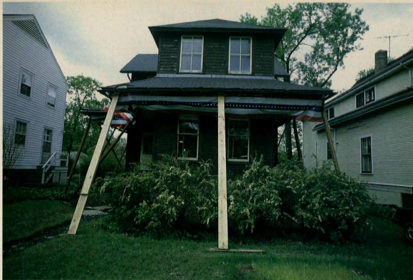
The rotted porch (above) was first to go during the dramatic renovation of Tom and Emily Hood's Winnetka, Ill., house (left).
