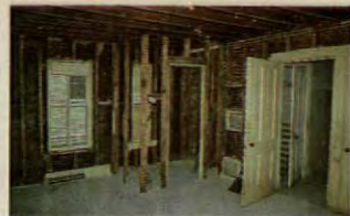
Inside, the Hoods stripped the kitchen bare. Joists came down to open the ceiling.
