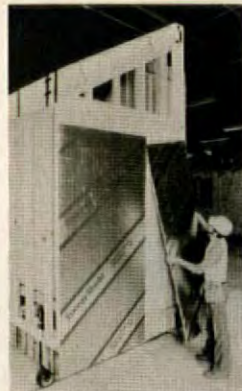
Outdoor living areas (left) and factory-installed insulation (above) exemplify NEST's quality design and construction.
