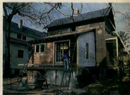
The rear kitchen, built circa 1900, gained a new south wall. The siding on the exterior is red cedar.
