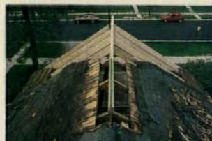
Added rafters on the front gable gave the old hipped roof a new peaked profile.
