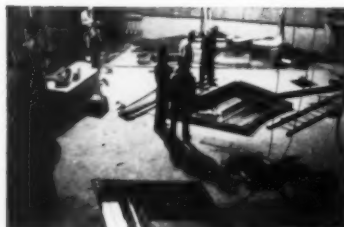
Pipes and wires are concealed beneath raised studio floor.
