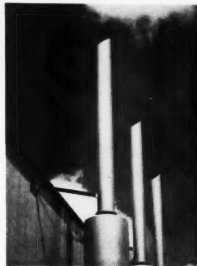
Diesel exhaust stacks painted with heat-resistant aluminum paint.
