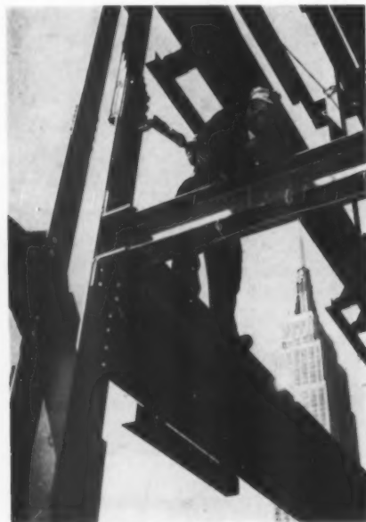
High strength bolts instead of rivets are being used in a new construction technique used by Anthony Campagna and Sons in the erection of an 18-story apartment building under the shadow of the Empire State Building. Not only is noise cut in half, but the two-man crew needs only a pneumatic impact wrench and holding wrench and no special scaffold.
