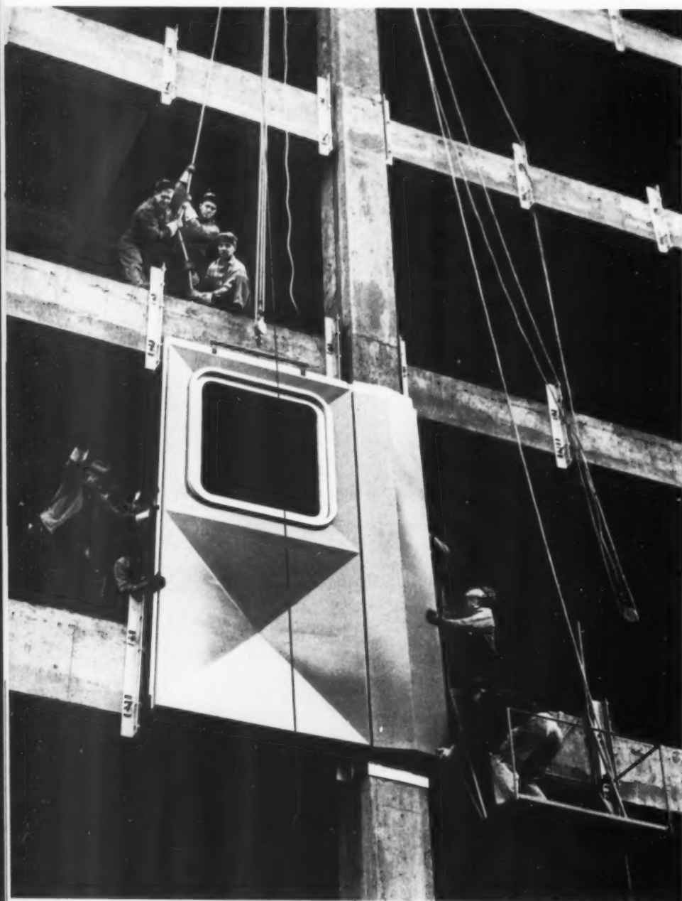
Wall panel being installed on the Alcoa Building. Architects Harrison & Abramovitz developed an encyclopedia of new uses for Alcoa's product (stair railings of aluminum cable, aluminum plumbing, etc.) and, most significantly, a prototype for some 300 aluminum-curtained buildings that have appeared since.
