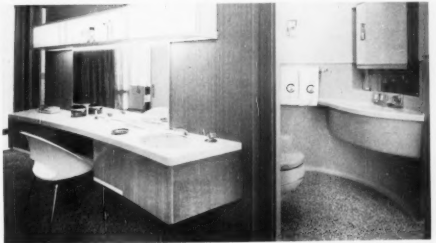
↓ Wall behind master bedroom vanity table encloses outer shell of adult's bathroom with its plumbing and heating connections. Elaborate vanity with lavatory is a major bedroom feature.
