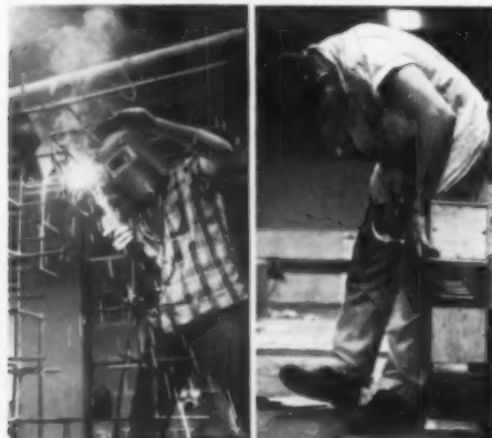
Construction of the full-scale exhibition was done entirely by students in Institute's shop.
