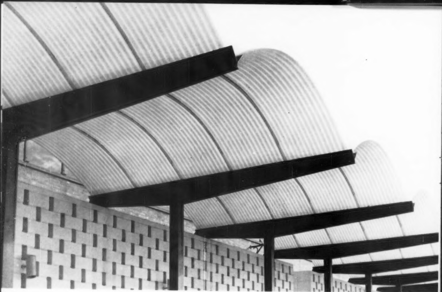
Corrugated canopy at Detroit's Willow Run Air Terminal. Molded by Structoglas Division, International Molded Plastics.
