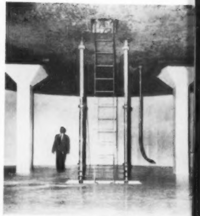
200,000-gallon underground storage tank for formaldehyde constructed of reinforced Laminac showed no signs of deterioration and no contamination of formaldehyde after 9 months of service.
