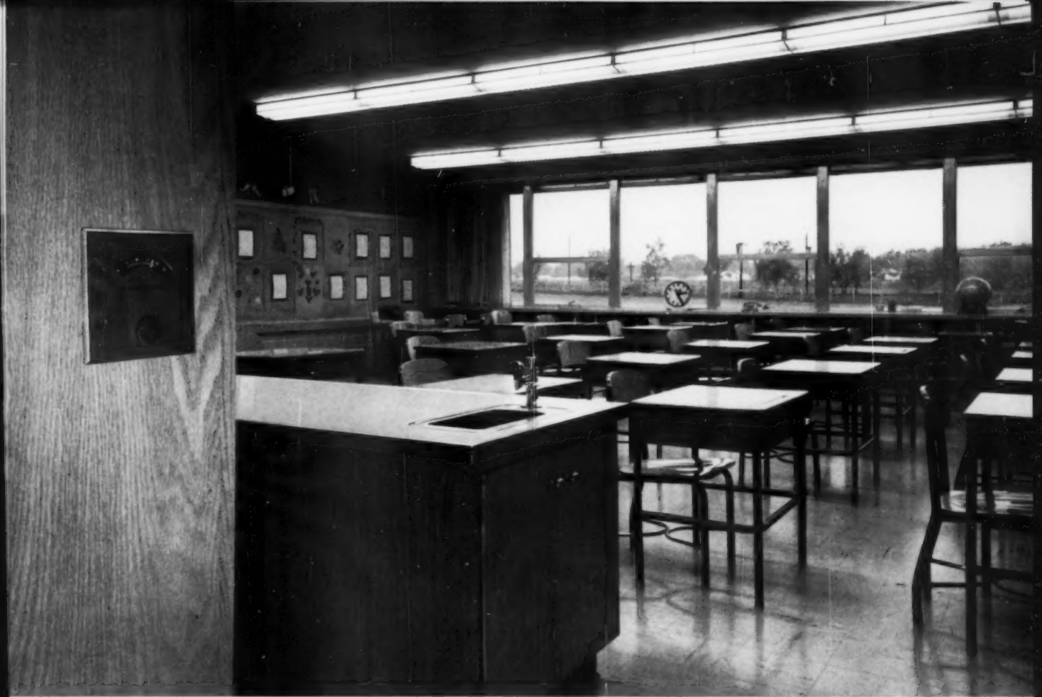
Automatic light control system includes a thermostat-like device which is set for amount of light desired. Control system measures amount of daylight entering room and dims or brightens artificial lights. (The Superior Electric Company.)
