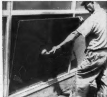
Faster glazing — installation of lights is done quickly and more efficiently when edges are protected by Butyl preformed gaskets.
