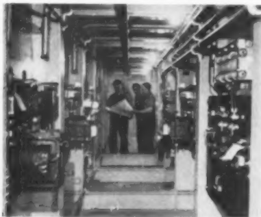
Interior of traveling crane
