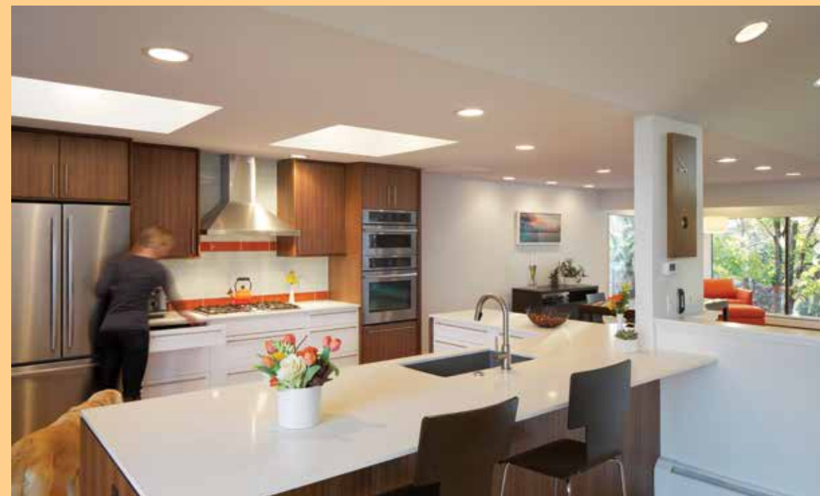
"The kitchen was completely enclosed," Jonas says. So his team took out two full walls. They added recessed lighting throughout the kitchen and even in the skylights in order to brighten things up.
