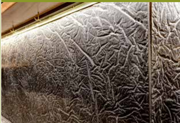
To create an organic texture on the front of the bar, Lujan and Blea "tried probably 100 different combinations of materials that we cast concrete against," before finally settling on a crinkled, shiny plastic that gave the concrete a unique textured quality. "We wanted it to be free-flowing, and to create shadow play and play up the light in the space," added Lujan.
