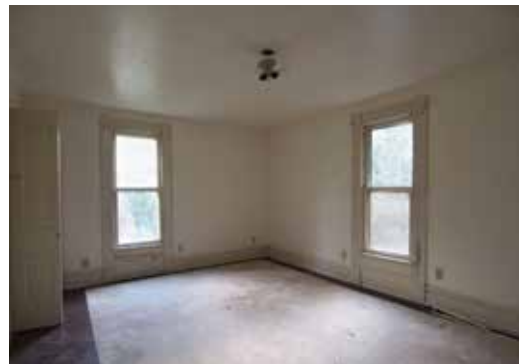
The original home's second floor had three bedrooms with flat ceilings. Arch11 quickly realized there was a great volume in the upper floors of the gable ends of the home and chose to integrate the attic space into the second floor. This design move allowed the interior to be informed in part by the exterior while creating a bright, serene living space among the treetops.
