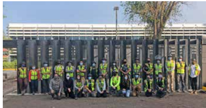
CBW students engage in the physical construction of the entire building. From tying the rebar and placing the concrete to installing the steel and CLT roof. The 2020 Colorado Building Workshop design-build cohort persevered through numerous COVID-19 delays and restrictions.
