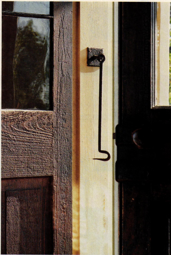
Salvaged French doors weathered by time add the patina of age, with much of their original glass and narrow wood muntins still intact. Antique box locks painted with a traditional coating of black asphalt are mounted on the face of the doors.
