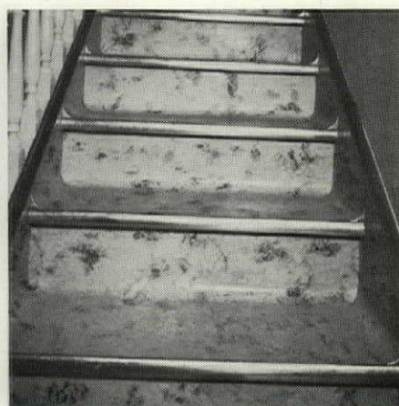
The sanitary aspect of this type of stair tread installation is readily evident. The linoleum used here is flashed up the risers and skirtings of each step in a single piece.
