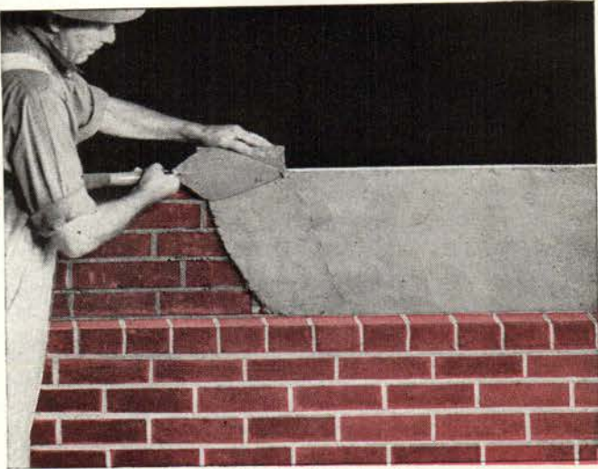
The face brick should be backplastered.
