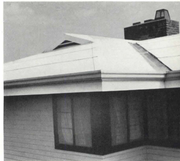
Photo of typical ridge, hip, and valley of plywood roof for residence on Fisher's Island, New York (above). Architect: Edwin D. Thatcher, New York. Detail drawings (left).
