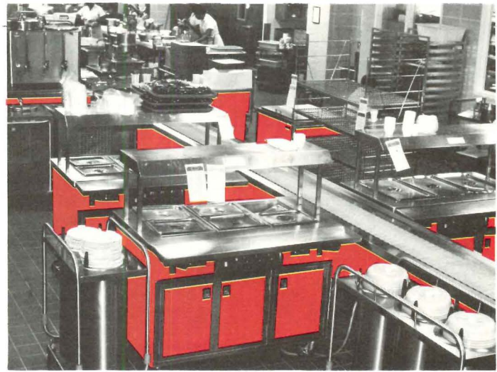
One solution to problem of "boiler room" aesthetics in the institutional kitchen is to dress up the tray make-up areas with colored fiberglass.
