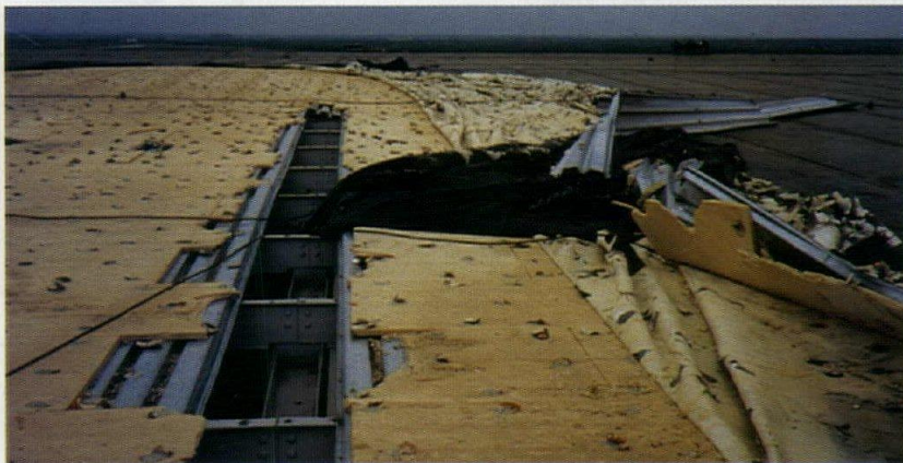
1 An adhered roof system exposed to high winds has delaminated at the insulation facers.
