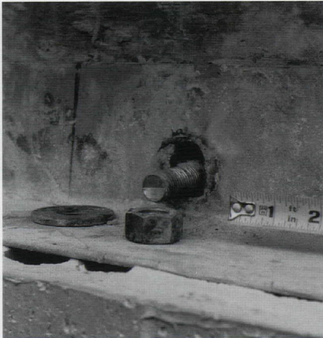
5 BOLT HOLE ENLARGED WITH A BLOW TORCH
