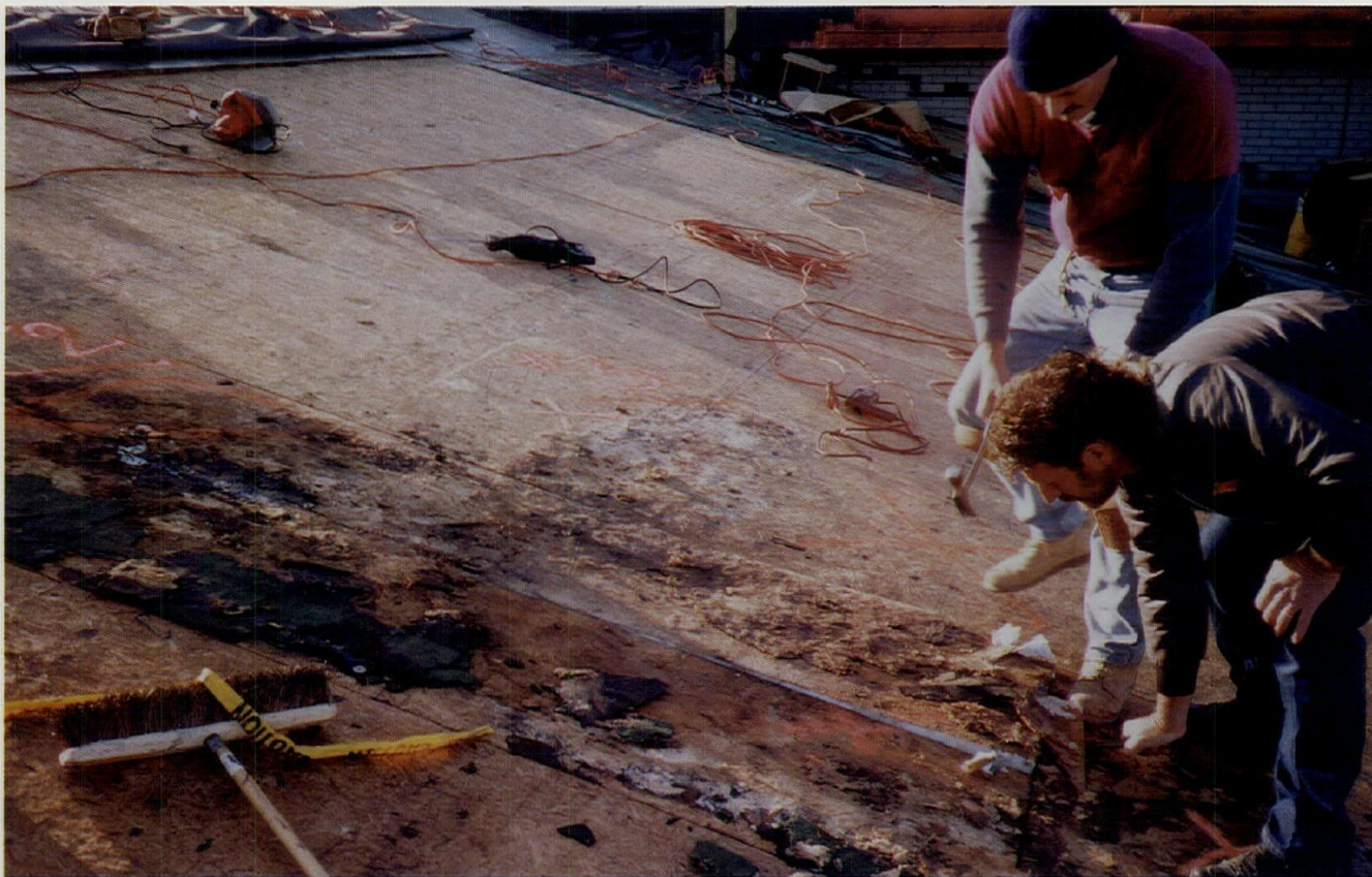
7 DEGRADED AND DEFLECTED ROOF DECK PANELS
