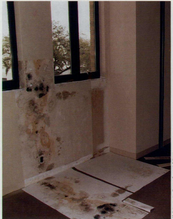
1 MOLD GROWTH BEHIND VINYL WALL COVERING
