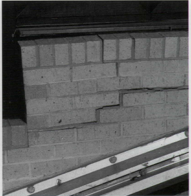
6 BULGING CONCRETE VENEER AT WALL-ROOF INTERSECTION
