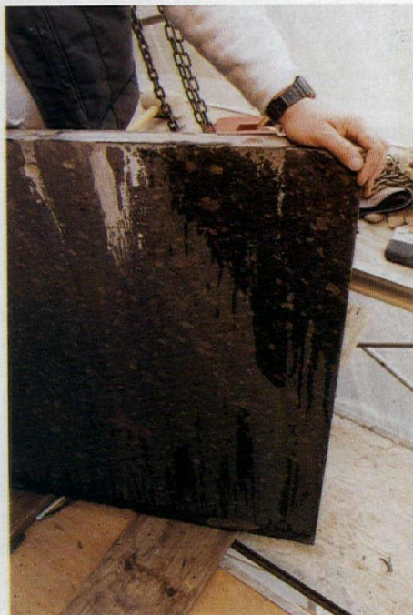
Frozen exfiltrating water vapor from a skylight system incapable of supporting the interior humidified environment (1). Granite cladding shows exfiltrating water vapor condensing on its interior surface (2).
