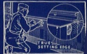
The outer edge of inner member serves as a true, unvarying line to which face of structural material is set.
