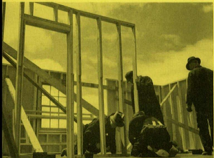
Dividing partitions assembled in sections at the mill are then put in place ready for Sheetrock Wallboard.
