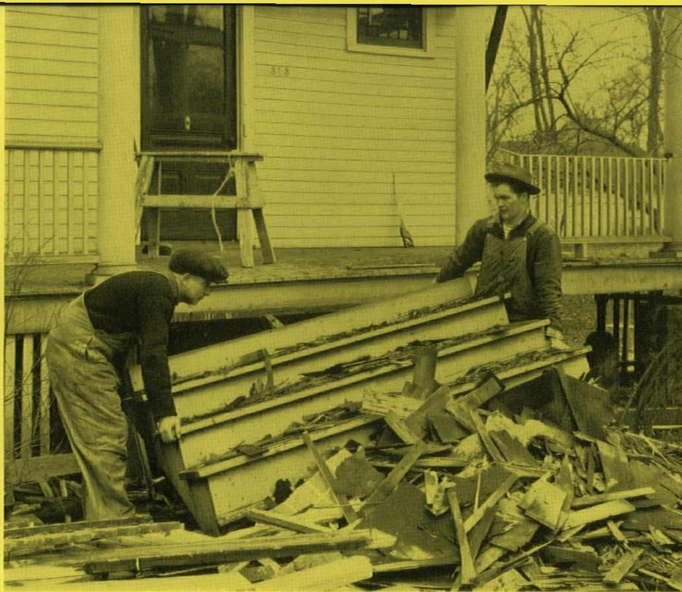
Removing old style porch from USG Research Remodeling House. Eugene Voita, Chicago, Architect.
