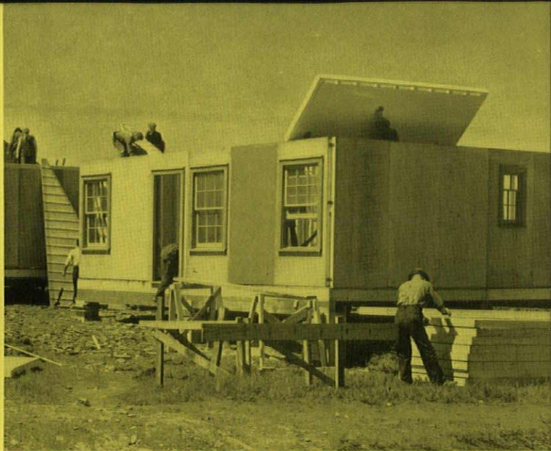
The ceiling panel with Sheetrock attached is placed in its position on top of the walls and dividing partitions.
