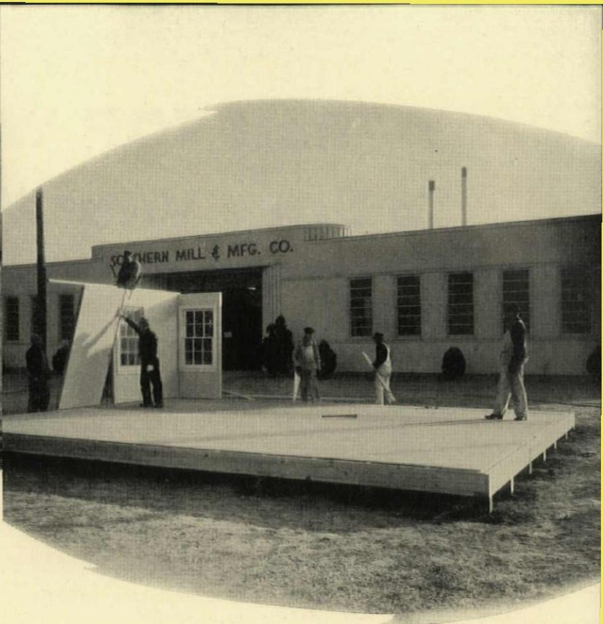
Exterior wall panels locked in place at sill, plate and vertical joints; note perfect alignment of Sheetrock surfaces.
