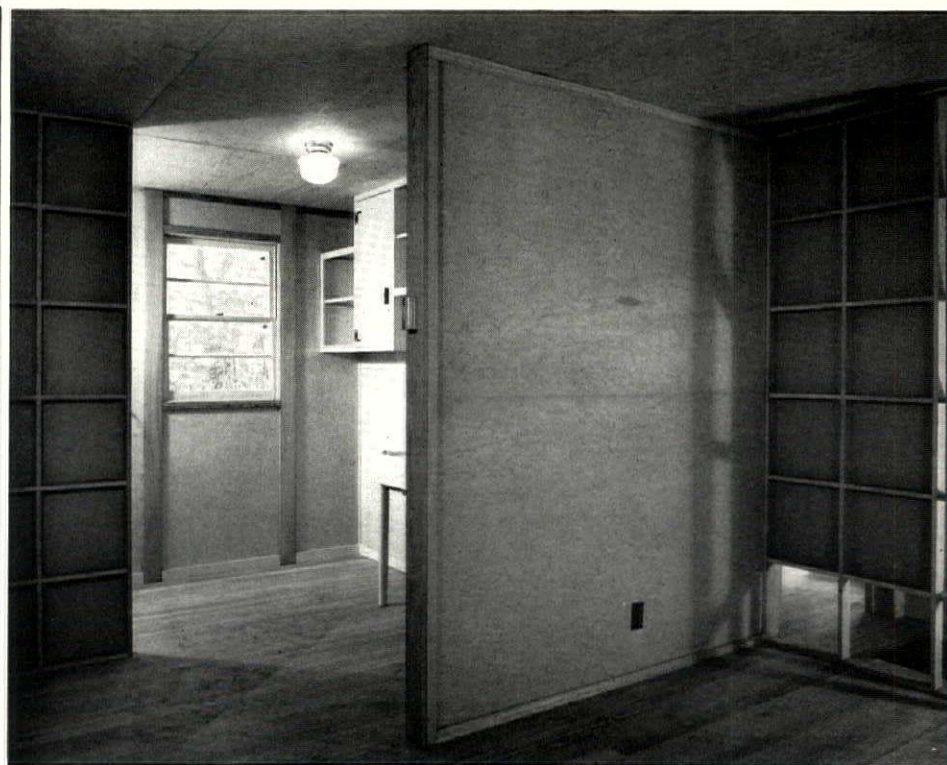
Interiors show the "egg-crate" construction of the wall panels, and provision of built-in furniture.
