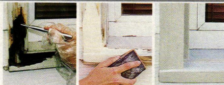
Restoration of rotted window is easy and cost-effective.
