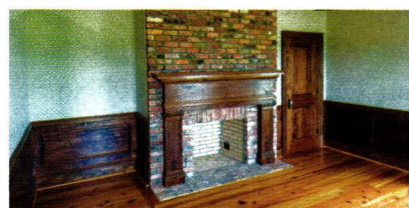
Drivood provided the wood mantel for this old South Carolina vernacular farmhouse outside of Darlington, SC.
