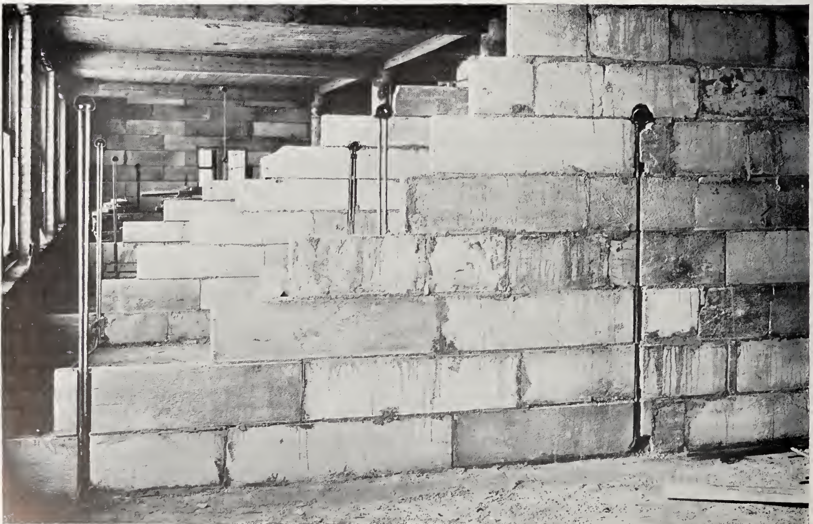
CONDUIT AND OUTLETS FOR ELECTRIC LIGHT WIRES IN PARTIALLY COMPLETED MACKOLITE PARTITIONS.
