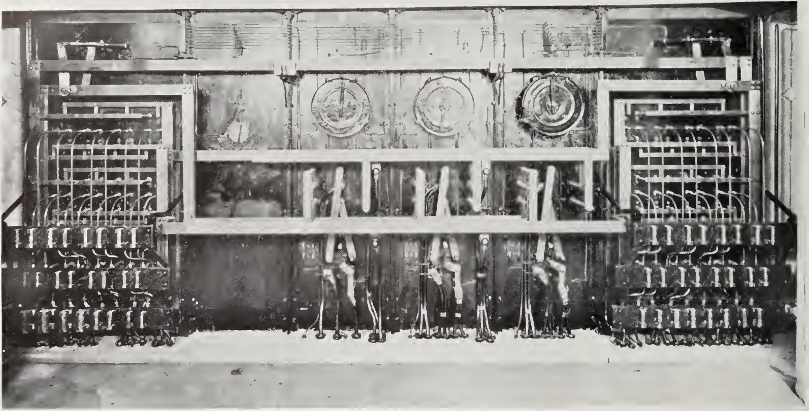
REAR OF GENERATOR AND FEEDER PANELS OF MAIN SWITCHBOARD.
