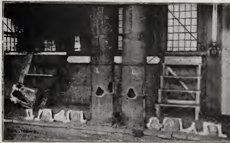
Fig. 11.—Fracture of Brackets on 15-in. Columns, B2, I and II.
