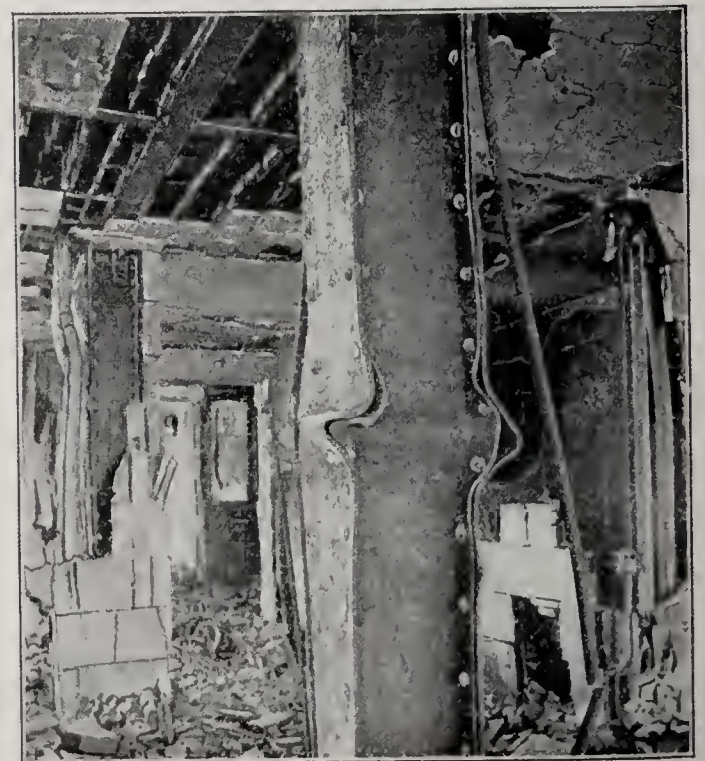
Steel Column on Seventh Floor, of the Calvert Building, Baltimore, Md' Buckled by Heat through the Loss of its Protecting Covering. Carpentry and Building.
